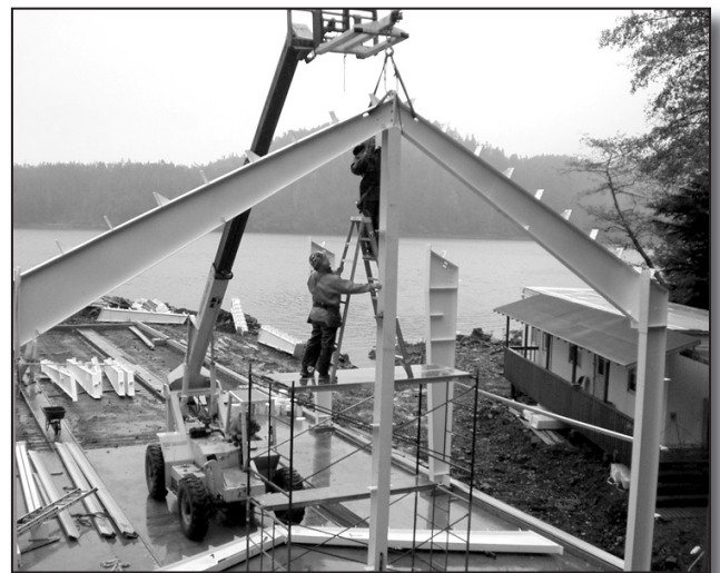
North Star Construction erected our new incubation building, funded by the chum Southeast Sustainable Salmon Fund (SSSF) grant.
